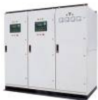
DSE-550 Parallel Control Panel system
